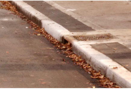
Figure 3.56 A side inlet catch basin
